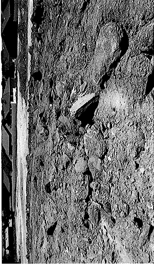
Figure 4 – Problematic shale gradation, large hard block too few of fines
